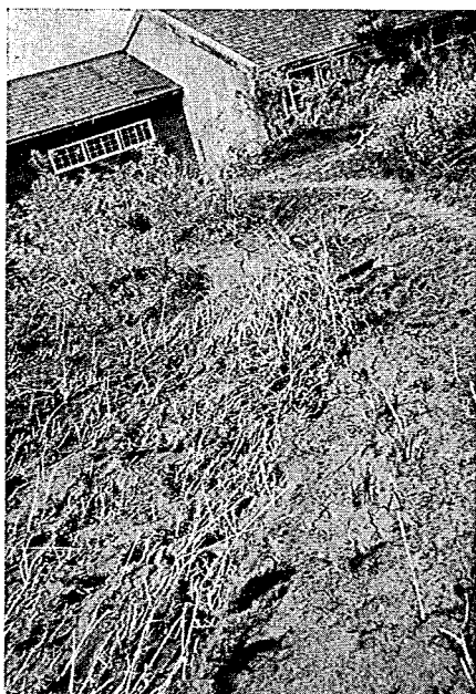
Photo 10 Landslip. A hill at the back of Ken'yoshi middle school in Sannohe town. 剣吉中学（三戸）裏の山くずれ
