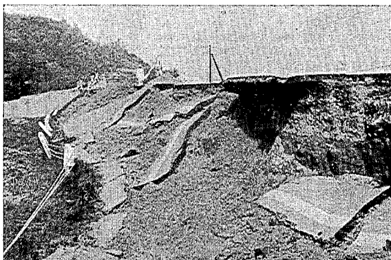
Photo 4 Slope failure of embankment at Kitataikaiwa, Fukuji village, National Highway Route 104.
