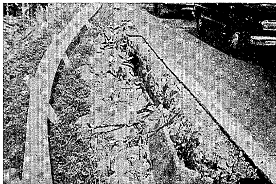
Photo 2 Failure of shoulder near Takayashiki, Shiroishi town, National Highway Route 45.
