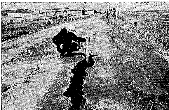
Photo 20 Cracks on the embankment of the Mabechi River at a distance of 400 meters from the river mouth.
