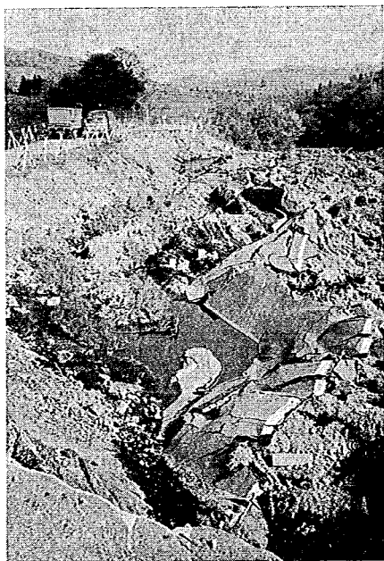
Photo 1 Damage of banking (Metoki area of Route 4).
