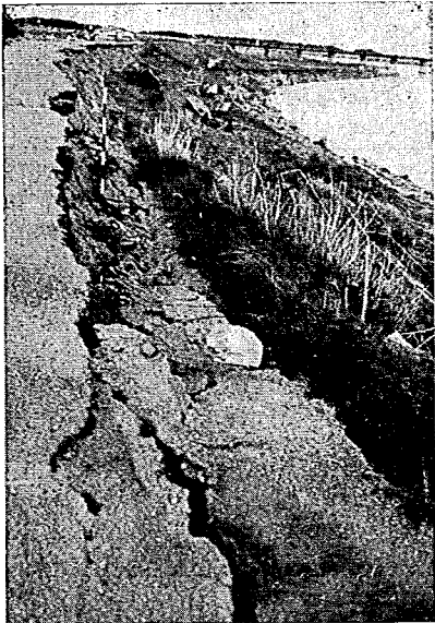
Photo 19 Cracks and failure of the side slope on the embankment of the Aisaka River at Horikiri.
