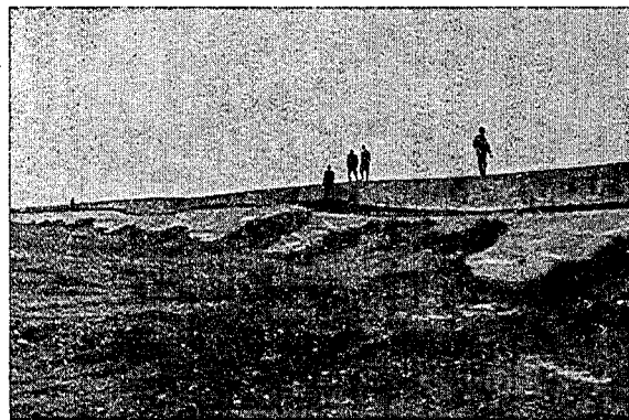
Photo 26 Ununiform settlement of the coastal dike at Momoishi. 百石海岸堤防の不等沈下による天端高の不整
