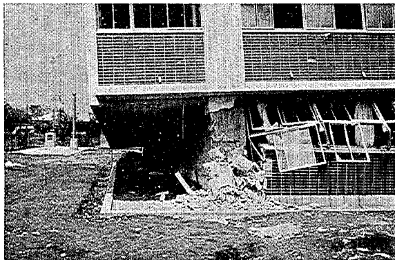
Photo 23 Damage of reinforced concrete building (Misawa commercial high school in Misawa city). Enlarged photo of the part of collapse. 三沢商業高校校舎の被害，座屈した部分
