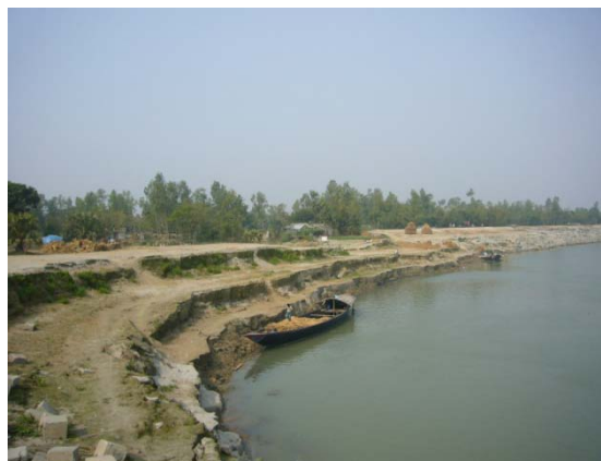
Photo 6-30 The jetty's foundation was considerably eroded.
