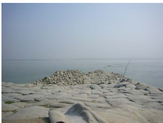
Photo 6-29 A jetty whose tip had been washed out
