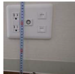
Electric outlet and modular jack with slots 20cm from floor
