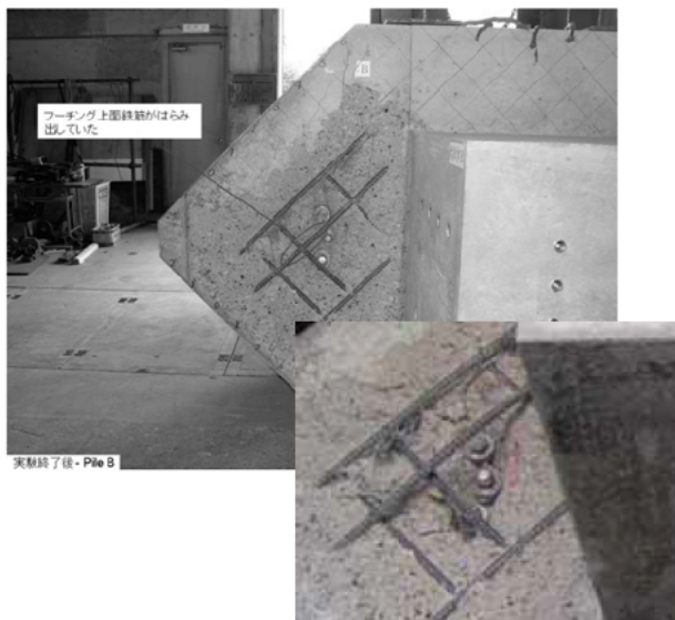
杭の鉛直押抜きせん断破壊 (c) Case SPP-C-1
