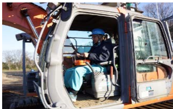
Fig.C-7 Boarding operation using the remote control device
