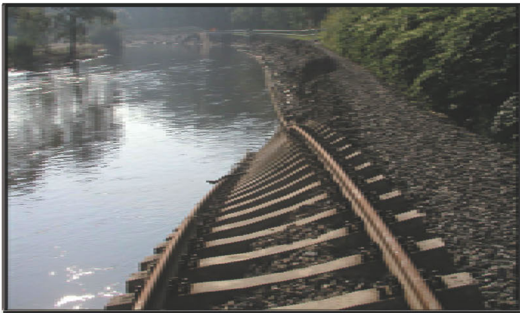
Figure 7 Typical damage to the railroads: Zschopau river (branch of Mulde)
