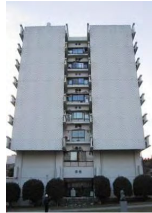
Photo 3.32 Appearance of Damaged Building
