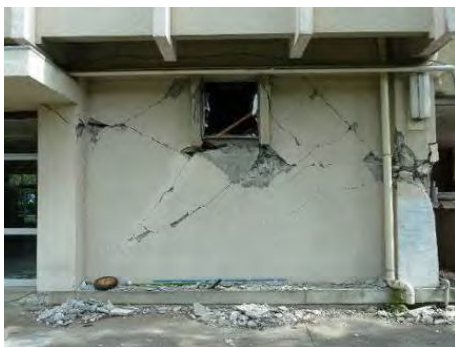
Photo 3.27 Shear Failure of Wall with Opening
