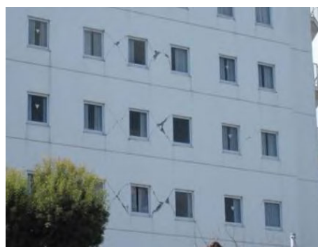
Photo 3.42 Shear Crack on Nonstructural Wall
