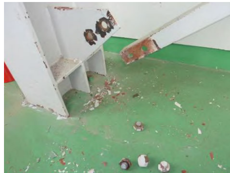
Photo 3.50 Fracture of Bolts
