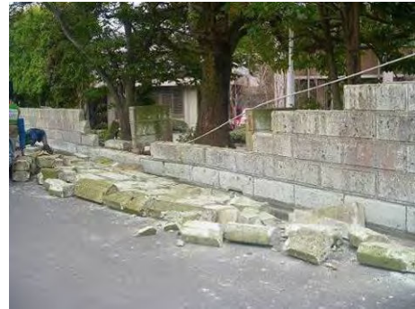
Photo 3.46 Collapse of Stone Masonry Wall
