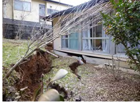
Photo 3.9 Damage of House
