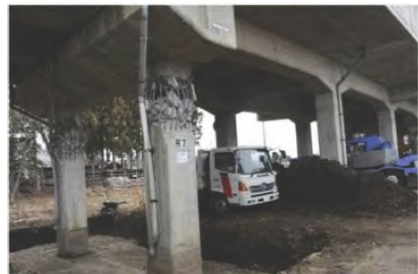
Photo 16 Damage of R7 column, No. 1 Nakasone viaduct during 2011 Great East Japan earthquake
