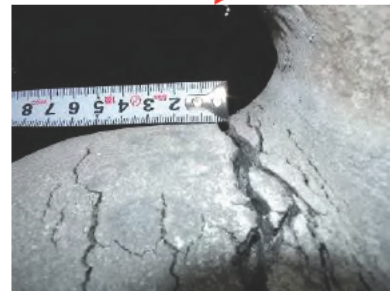
Photo 3.77 Lead Damper and Crack on the Surface
