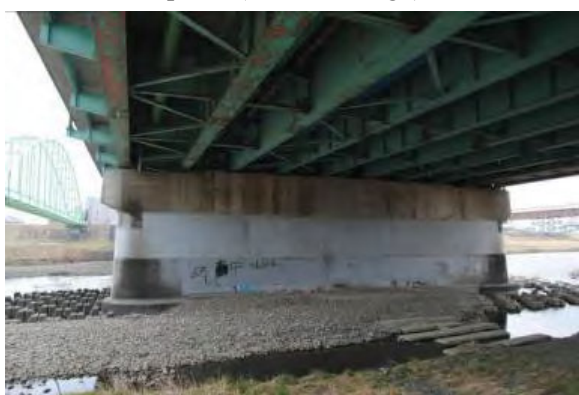
Photo 7 Retrofitted pier of Sendai Bridge which did not suffer damage during 2011 Great East Japan earthquake
