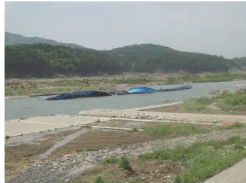
Fig.4(2) Wash Away of Steel Girder of Koizumi Ohashi Br. (June 4)
