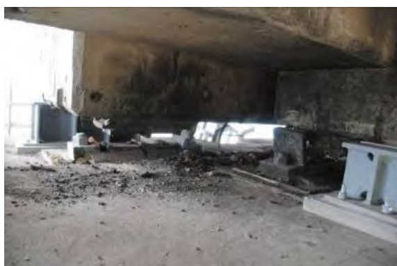
Photo 3 Damage of pin and roller bearings
