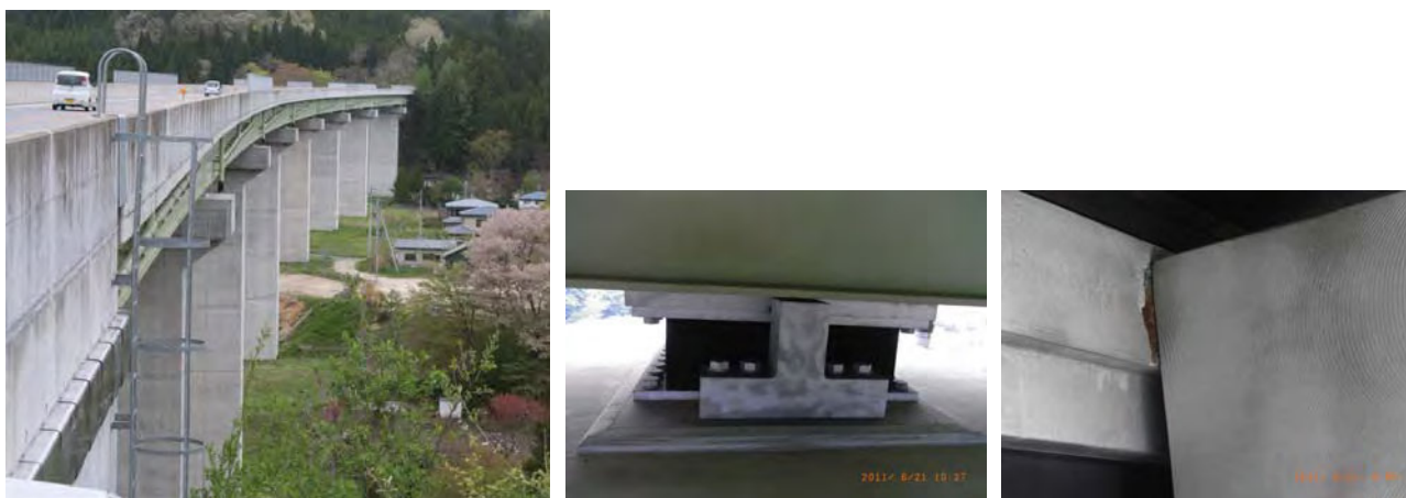
Photo 3 Yamada viaduct and its bearing. The top plates of bearings were scraped by the side blocks.
