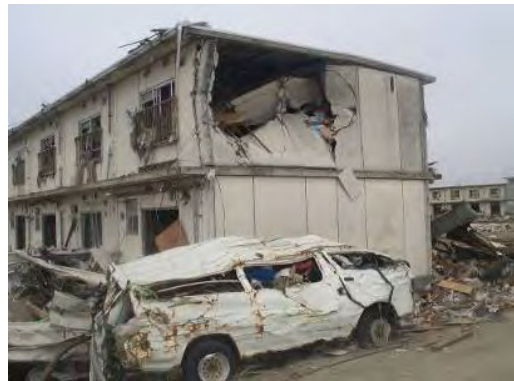
Photo 4.6 Wall Opening Generated by Debris Impact
