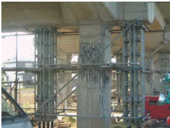
Photo 14 Shear failure of RC columns at Odaki viaducts after 2003 Sanriku-Minami earthquake
