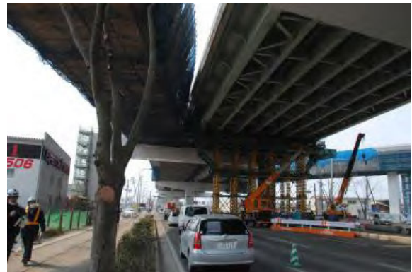
Photo 10 Piers where elastomeric bearings ruptured (Sendai-Tobu viaduct)
