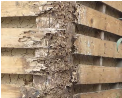
Photo 3.13 Bio-deterioration of Column and Based Mortar
