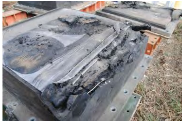
Photo 12 One of elastomeric bearings ruptured
