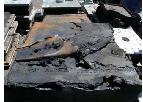
Fig.8(4) Rupture of Rubber Bearing (April 6)
