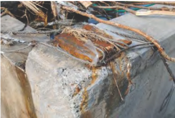
Photo 22 Failure of a RC side stopper, and four steel stoppers for preventing excessive longitudinal deck response which were not damaged
