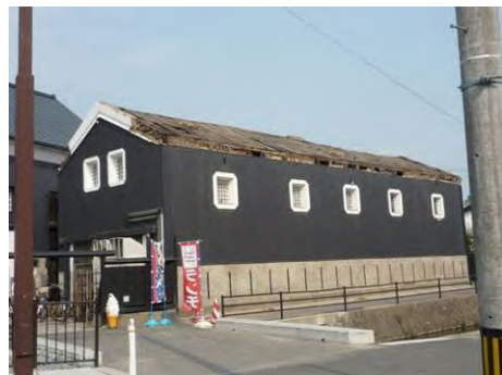
Photo 3.5 Warehouse with Mud Walls whose Roof System with Roof Tiles fell down
