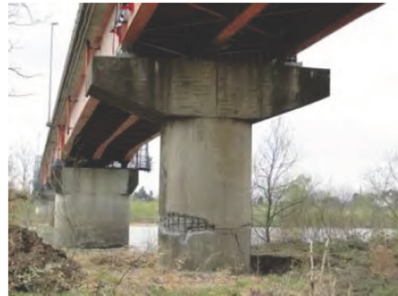
Photo 1 Shear failure of a column due to termination of longitudinal bars with insufficient development (Fuji Bridge) (courtesy of Dr. Hoshikuma, J., PWRI)
