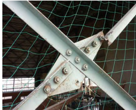
Photo 3.48 Net Section Fracture at Bolt Hole
