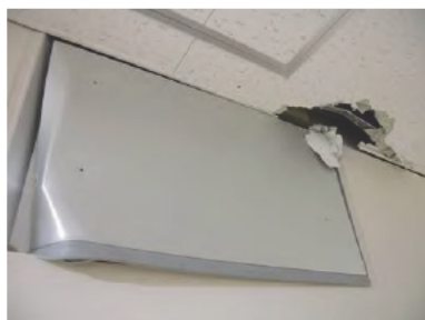
(a) Damage to the panel
