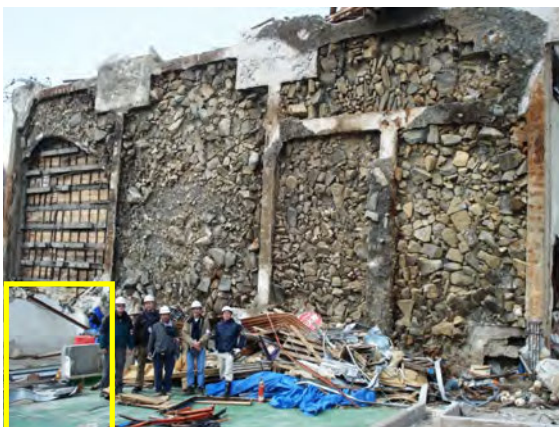
Figure 3 The ASCE Tohoku Tsunami Reconnaissance Team at the Onagawa uplifted and overturned 2-story reinforced concrete cold-storage building - Note low wall with top edge spalled (Hideyuki Kasano)
