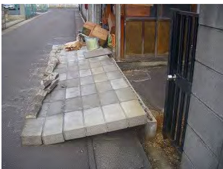
Photo 3.45 Collapse of Concrete Block Wall
