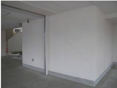
Photo 3.74 Shear Crack on the Wall
