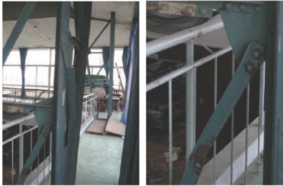
a) Latticed column b) Buckling of diagonal member Photo 3.51 Buckling of Diagonal Member of Latticed Column
