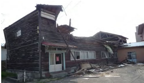
Photo 3.7 School Building whose 2 nd Story Collapsed
