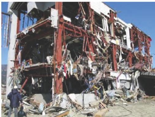
Photo 4.12 Remaining 3-story Steel Building
