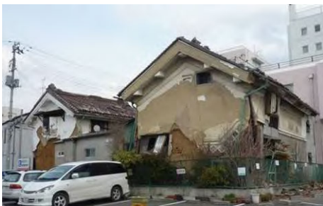
Photo 3.14 Dozo with Residual Deformation
