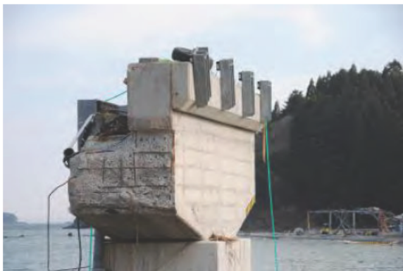
Photo 23 An upper steel bearing after damaged
