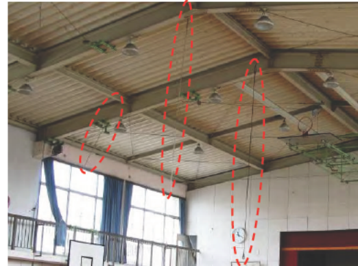
Photo 3.53 Fracture of Horizontal Brace
