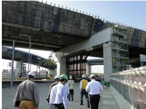
Fig.8(1) Sendai-Tohbu Viaduct (June 3)
