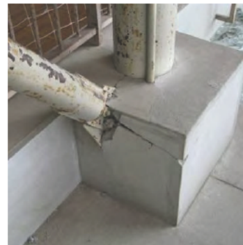
Photo 3.54 Cracking of Column Base Concrete
