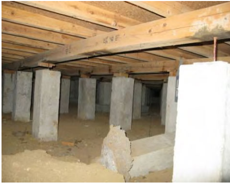
Photo 3.55 Overturning of Floor Strut
