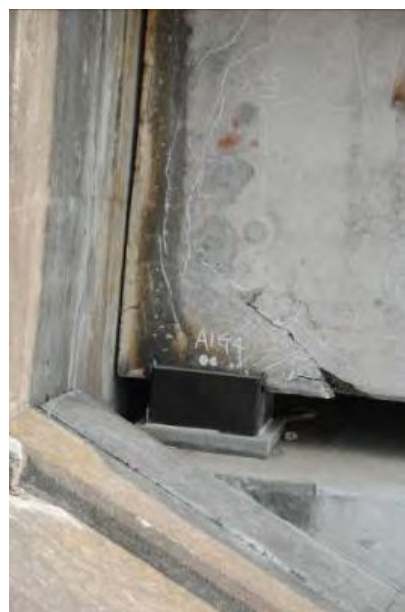
Photo 4 Damage of PC girders near the support
