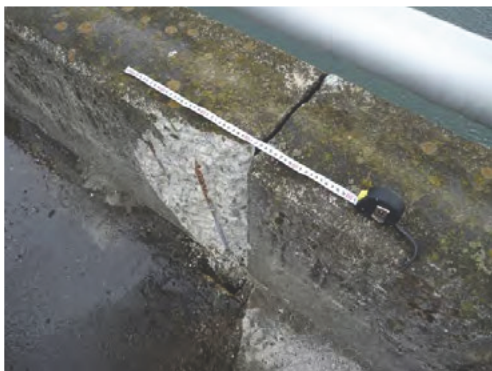
(a) Exfoliation of parapet concrete
