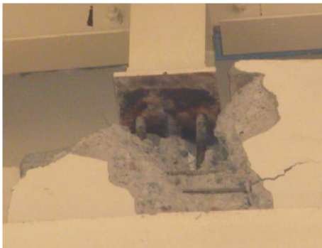
Photo 3.52 Spalling of Concrete
