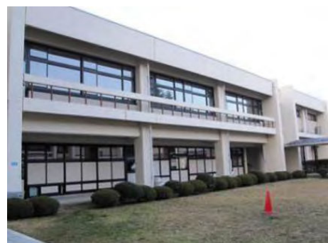
Photo 3.24 Appearance of Damaged Building
