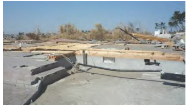
Photo 4.13 Remaining Ground Sill after Washout of Superstructure
