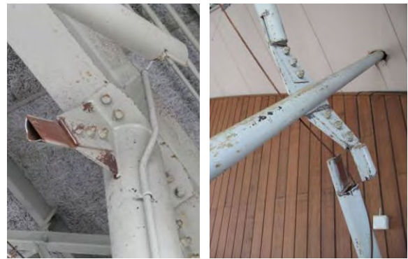
a) Fracture at column top b) Fracture at brace crossing Photo 3.49 Fracture of Brace Welded Connection
