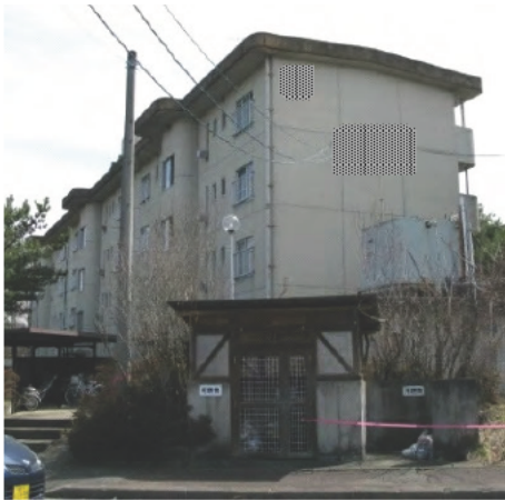
Photo 3.34 Appearance of Sank and Leaned Building
