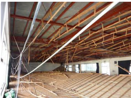
Photo 3.57 Dropping of Ceiling Materials
