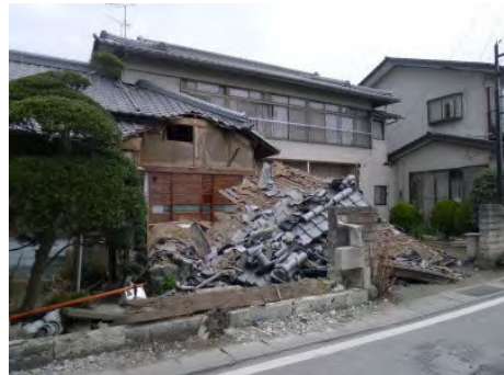
Photo 3.17 Breakage of Entrance Part
