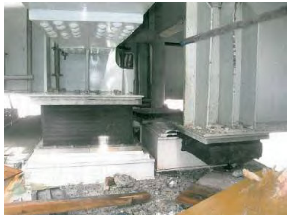
Photo 11 Transverse offset of a girder due to rupture of elastomeric bearings
