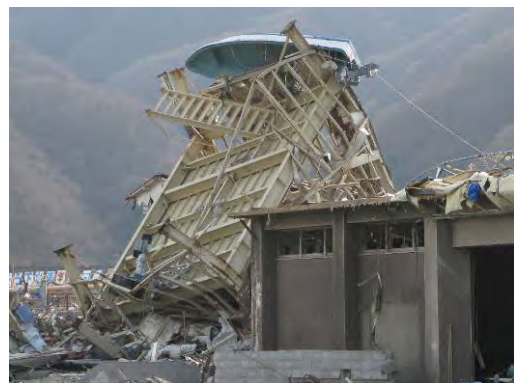
Photo 4.7 Steel Building Overturned by Fracture of Column Base Anchor Bolts
