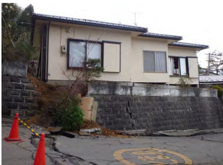
Photo 3.8 Damage of Retaining Wall and Houses (Oritate, Aoba Ward)
