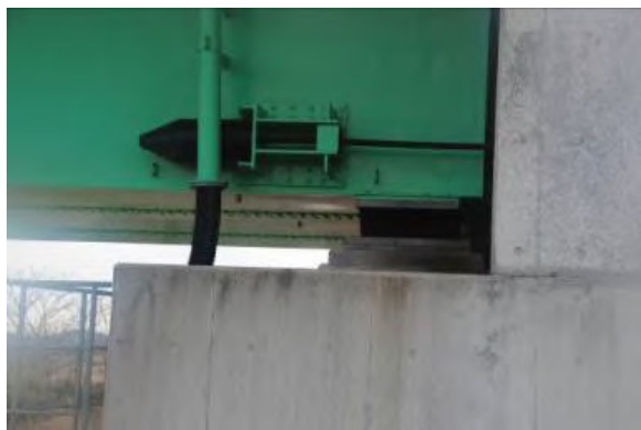
Photo 9 An end of deck supported by elastomeric bearings and unseating prevention devices
