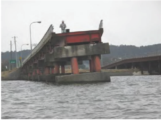
(a) Collapse of Bridge with Pile-bent Columns
