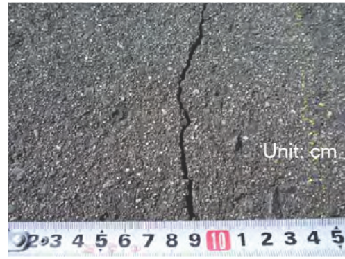
(b) Closeup of a crack
