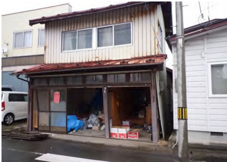
Photo 3.2 Damage of Houses with Store
