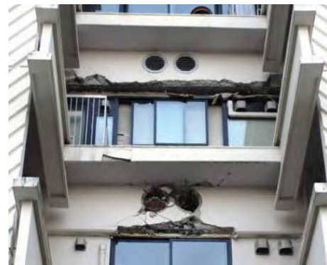
Photo 3.33 Damage on Boundary Beam with Opening
