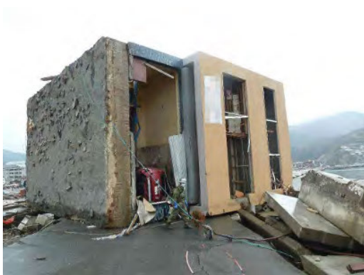
Photo 4.2 Overturning of 3-story Reinforced Concrete Building
