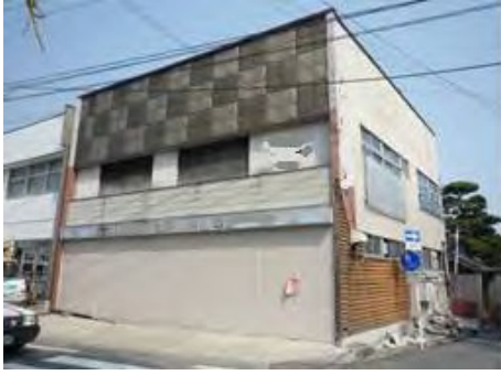
Photo 3.6 Store Combined House with Story Deformation
