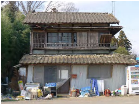
Photo 3.19 Damaged House with Shop
