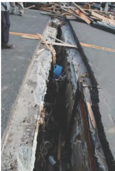
Photo 19 Effective restrainers to tie together adjacent decks
