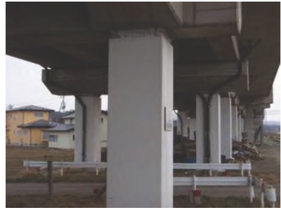
Photo 15 No. 3 Odaki viaducts which were retrofitted after 2003 Sanriku-Minami earthquake performed well during 2011 Great East Japan earthquake
