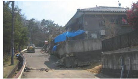
Photo 3.67 Damage of Retaining Wall and House Movement and Tilting by Sliding and Ground Transformation
