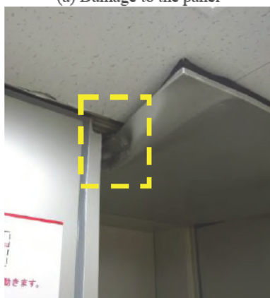
(b) Damage to the expansion joint
