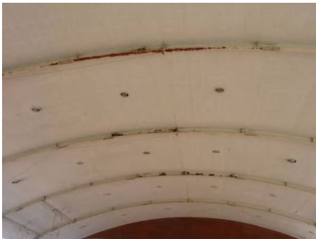
Photo 3.56 Peeling of Paints of Beam
