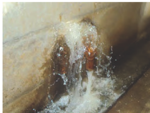
(b) Leakage from contraction joint 2J3
