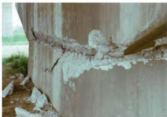
Photo 6 Damage of a pier during 1978 Miyagi-ken-oki earthquake (Sendai Bridge)
