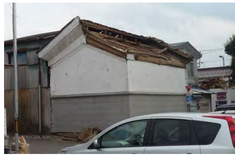
Photo 3.15 Fallen Roof Tile of Dozo
