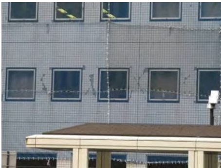
Photo 3.44 Damage of Tile on Exterior Wall
