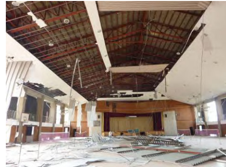
Photo 3.58 Dropping of Ceiling Materials
