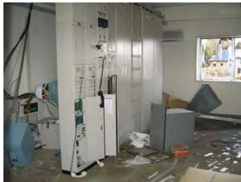
Photo 1 Data logger of KSN station that was attacked by tsunami.
