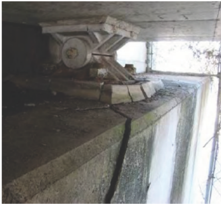
(c) Damage to Pier Top
