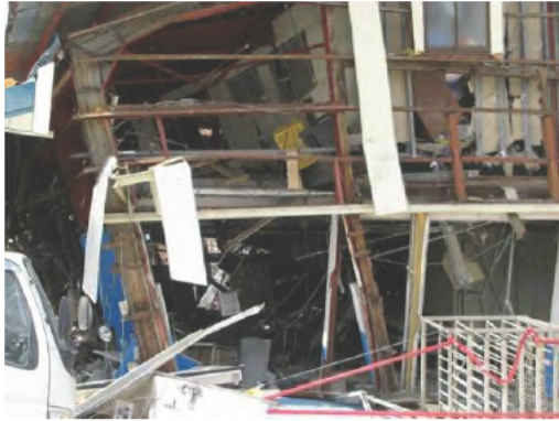
Photo 4.11 Tilted Gabled Roof Frame
