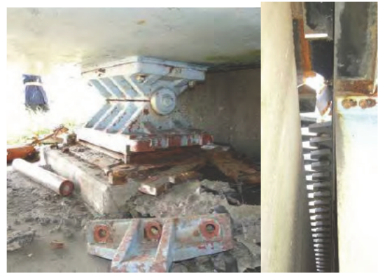
(d) Subsidence of Deck-End Resulting from Broken Movable Bearing
