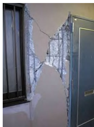
Photo 3.41 Shear Failure of Nonstructural Wall
