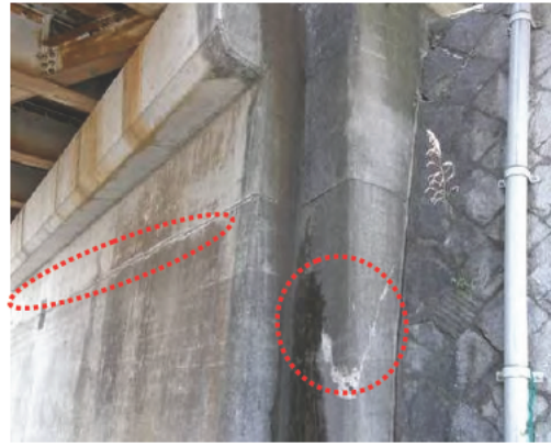
(b) Damage to RC Pier Wall with Small Amount of Reinforcement
