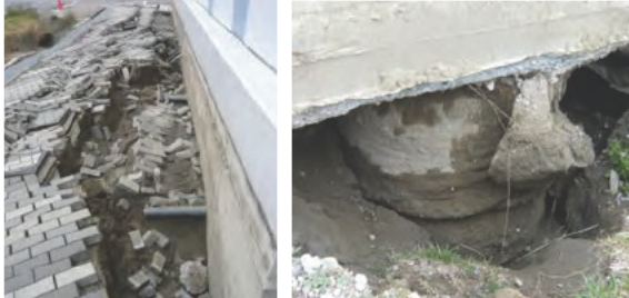
Photo 3.61 Situations around the Commercial Building and State of Pile Head
