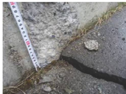
(b) Level difference at joint
