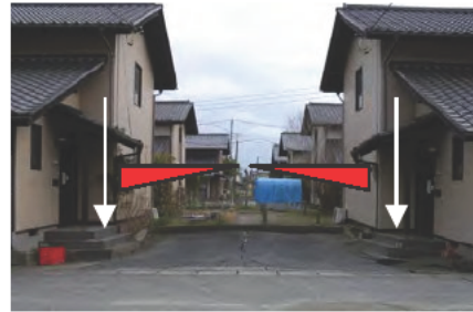
Photo 3.63 Subsidence of Two Houses enclosing Vacant Land
