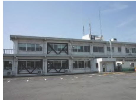
Photo 3.37 Appearance of Damaged Building
