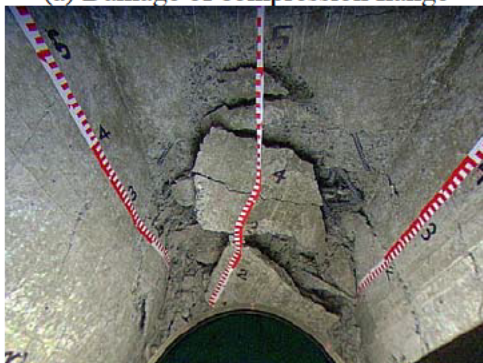
(b) Damage at inside wall
