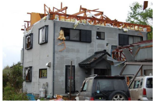
Photo 9 A damaged gable roof
