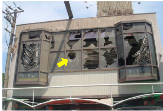
Photo 17 Damage to storefront glass
