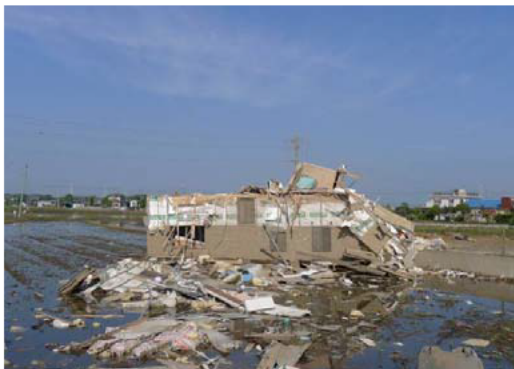
Photo 1 Wooden structure overturned from its foundation
