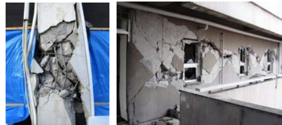
Fig. 23 Structural and non-structural damage of local government building
