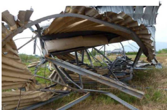
Photo 12 Collapse of Steel-frame building
