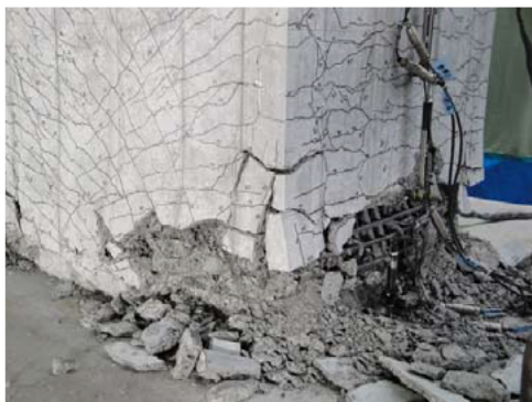
(a) Damage of compression flange
