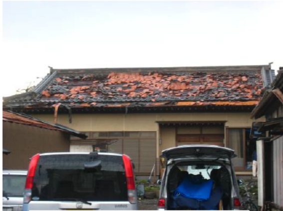
Photo 14 Displaced roof tiles
