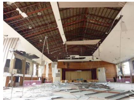
Fig. 5 Fallen down of ceiling
