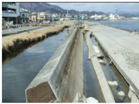
Photo 3.2 Seawalls collapsed toward the landside
