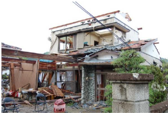
Photo 8 A damaged gable roof
