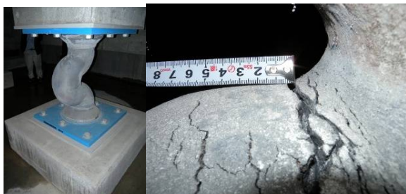
Fig. 8 Lead damper cracked
