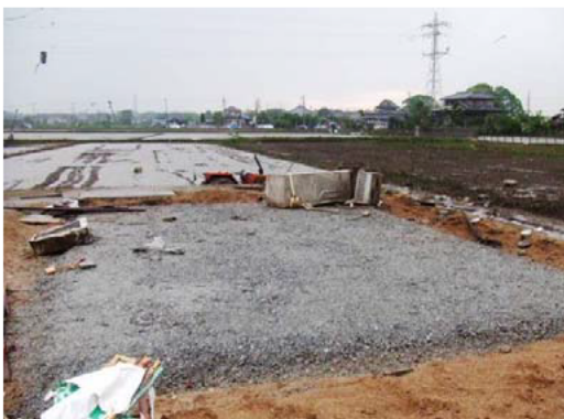
Photo 3 Condition of crushed stone under the foundation
