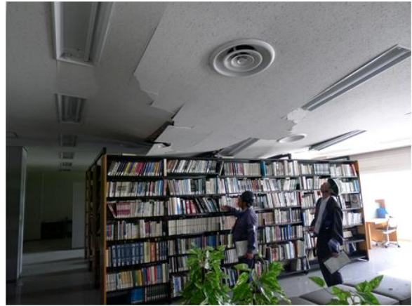
Photo 20 Damage to a ceiling
