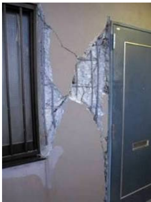
Fig. 7 Nonstructural wall failure
