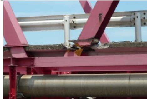
Figure 3 Fracture of Diagonal Bridge Bracing in Steel Truss Bridges
