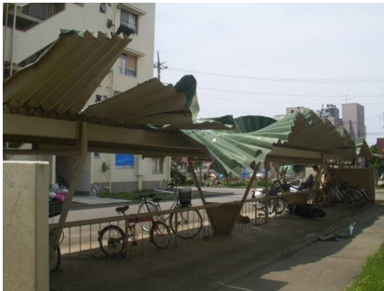
Photo 21 Remarkable deformation to the roof of a bicycle parking area
