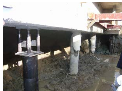
Fig. 24 Structural damage of pile head
