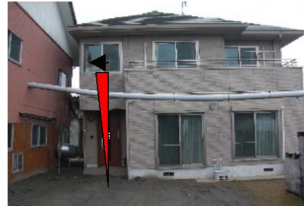
Fig. 9 Tilted house by liquefaction
