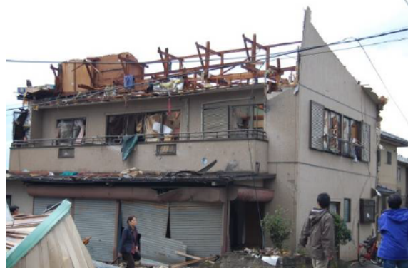
Photo 11 A damaged pent roof
