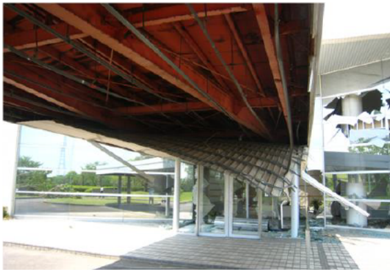
Photo 16 Finishing materials torn off the underside of an elevated walkway
