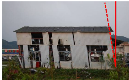
Photo 13 Residual deformation of Steel-frame structure
