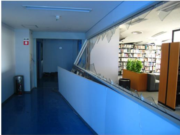
Photo 19 Damage to interior materials
