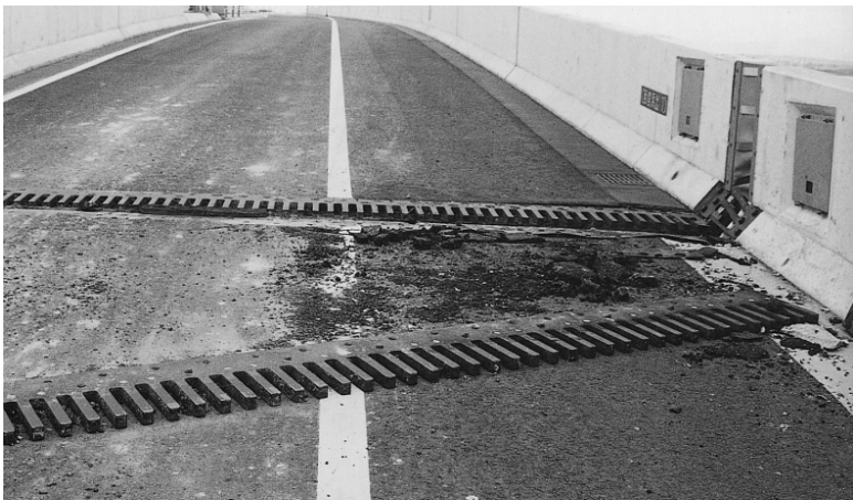
Photo 3.2.8 Damage of Expansion Joint
