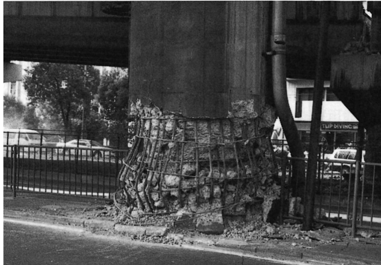
Photo 3.2.1 Bending Type Failure of Reinforced Concrete Columns
