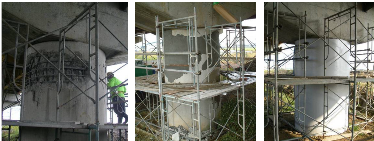
(a) Damage Situation
