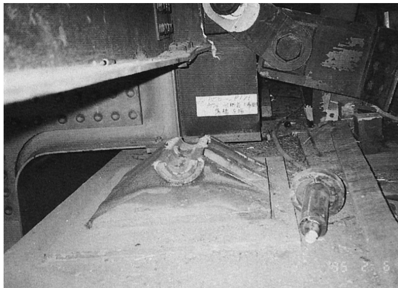
Photo 3.2.6 Damage of Pin Type Steel Bearing
