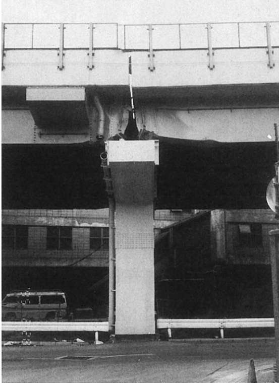
Photo 3.2.4 Damage at Ends of Steel Girders
