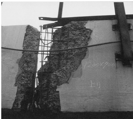
Photo 3.2.10 Damage of Safety Barrier for Vehicles
