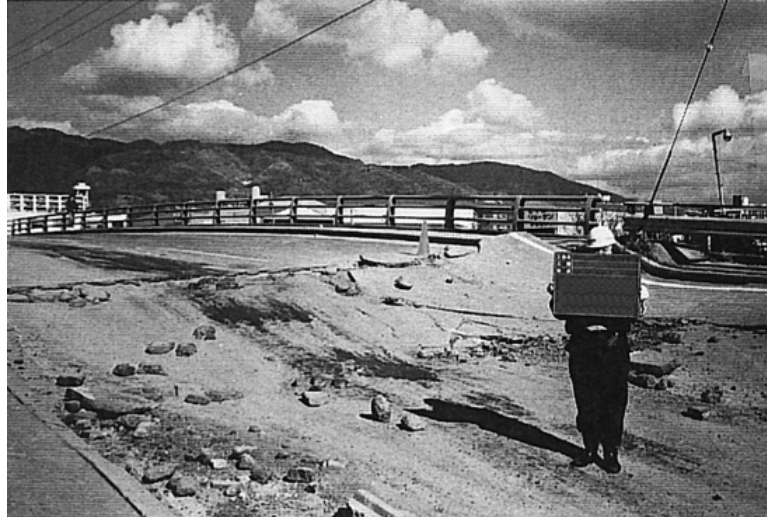
Photo 3.2.9 Settlement of Approach Section (Backfill Soil Section) of Abutment
