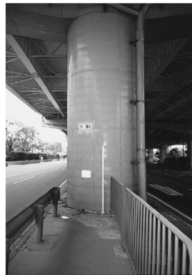
(b) Damage over the Ground
