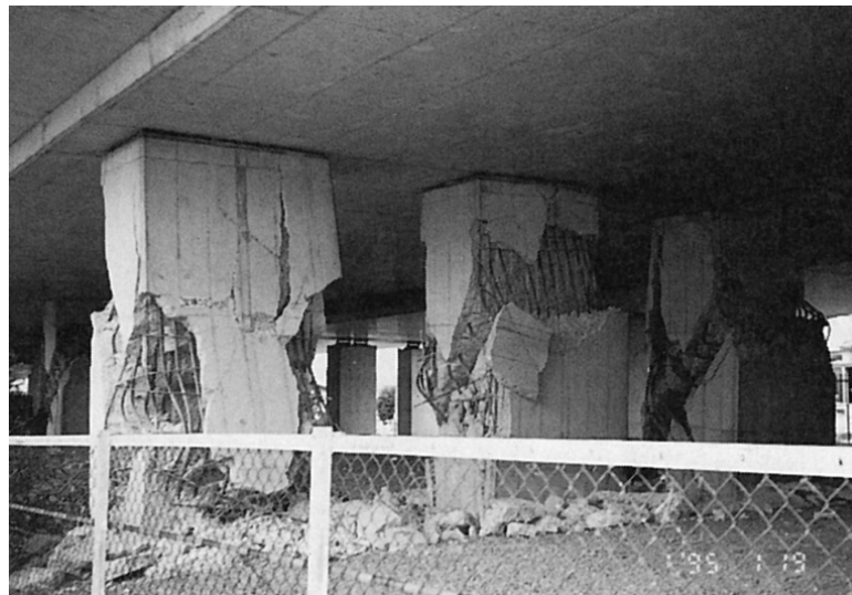
Photo 3.2.2 Shear Type Failure of Reinforced Concrete Columns
