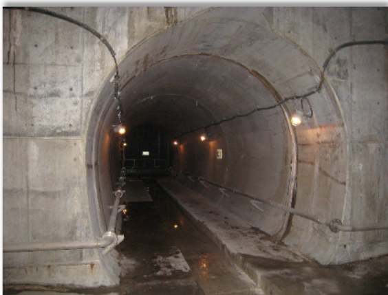
Onmawashi Park Underground Reservoir
